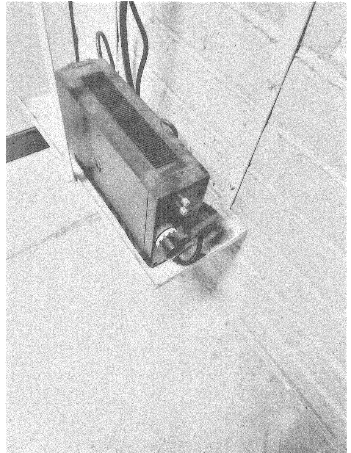
UNINTERRUPTIBLE POWER SUPPLY (UPS)
